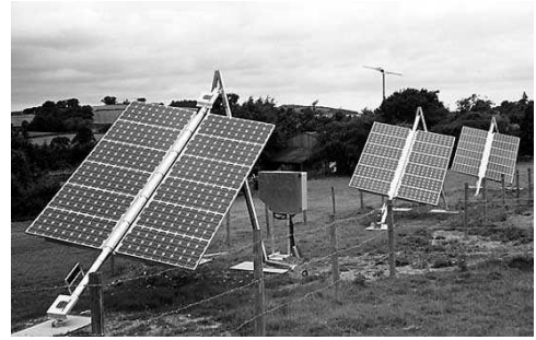
Fig.16 The solar pumping system 3 kW installed in Great Britain
