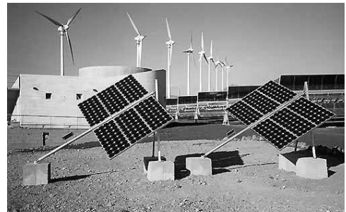
Fig.17 The solar tracking system 1 kW installed in Spain (Canaria Islands)
